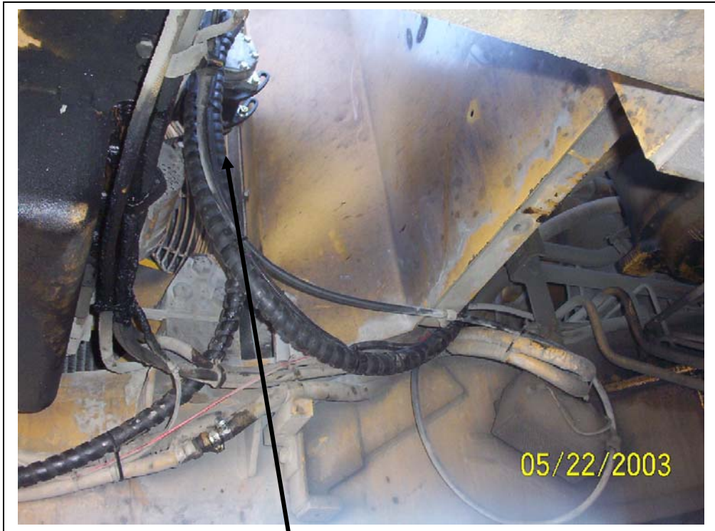
Hoses and wiring up to compressor.
